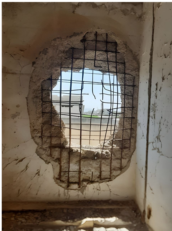
Figure 6. Severe Damage in the Load-Bearing Wall Caused by Direct Impact
