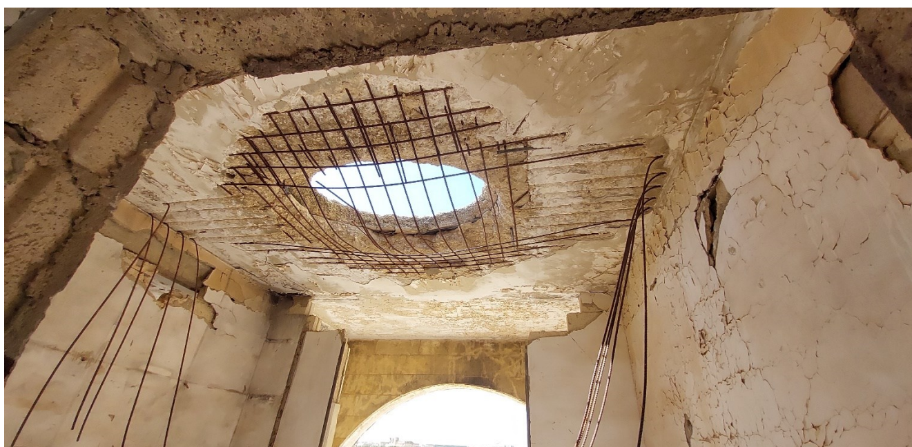
Figure 4. Structural Damage in the First-Floor Slab Showing Large Openings and Exposed Reinforcement
